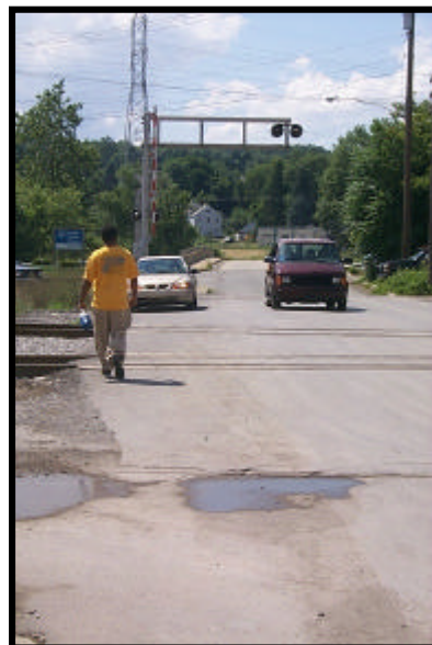
Figure 15. Poor pavement conditions along Clark Street (westward view).
